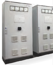
DC power 200kW for the air dual 800 A configurat to +55 ° C ambient tempe
