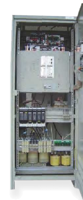
UPS System in a cabinet
