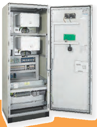
Hydroelectric power station, redundancy n+2
