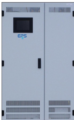
EPS/TSDCR Load system Regenerative
